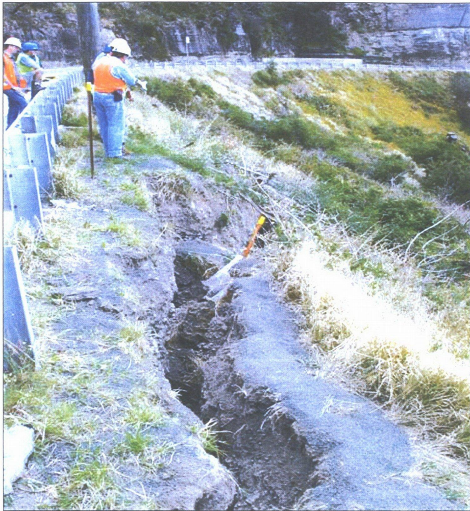
Plate 9.5: Current Embankment Failure GD2, July 2003
