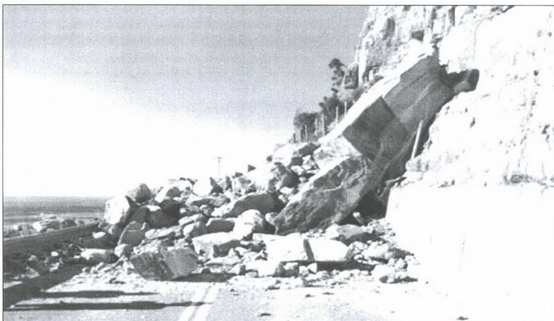
Plate 9.2: Plate 9.2 Major slab failure in 1987 (source RTA)
