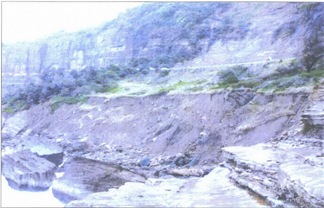
Plate 9.3: July 2003 Embankment Failure (Source: RTA)
