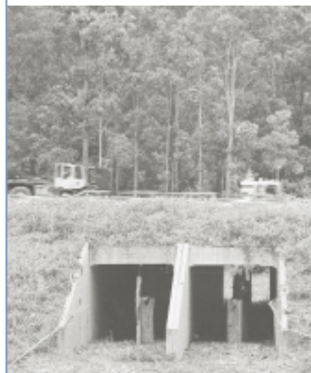
Fauna underpasses provide safe passage for animals beneath the Pacific Highway and include a raised structure to help protect climbing animals.
