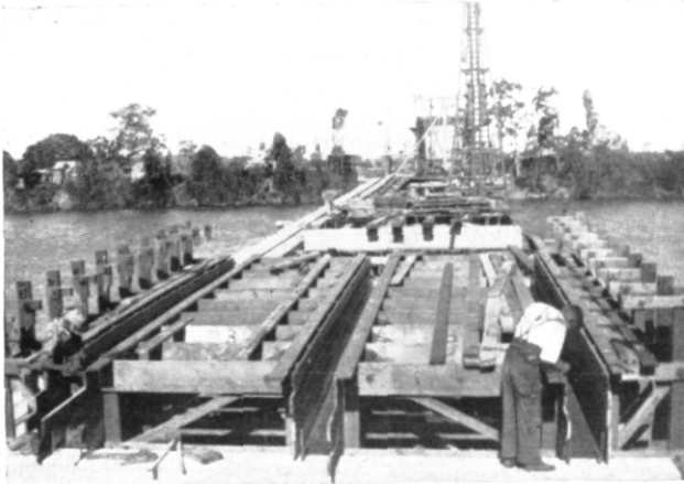
Frames for a three-girder bridge superstructure.
