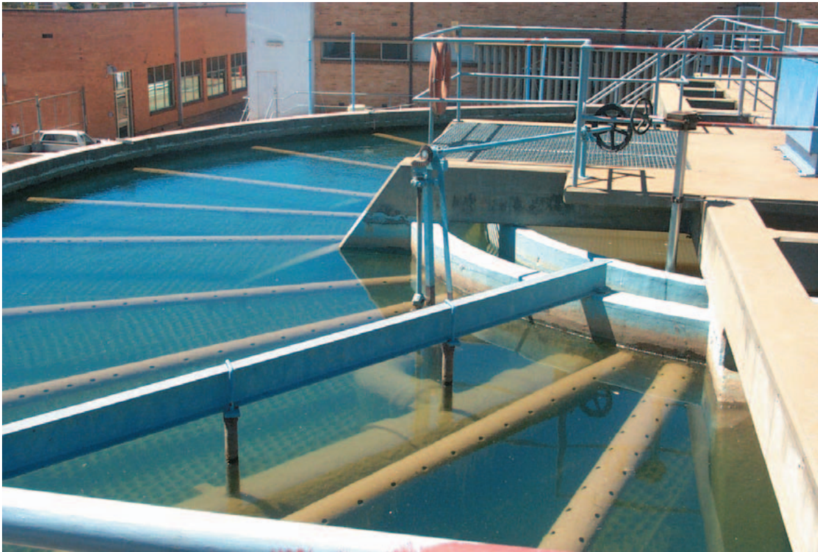
A clarifier at Mildura's 7th Street water treatment plant
