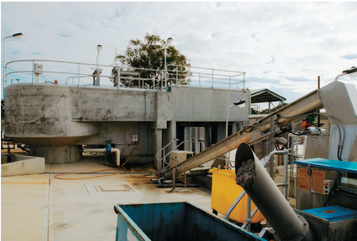
The new Kurri Kurri wastewater treatment works is catering for growth in the Coal Fields area
