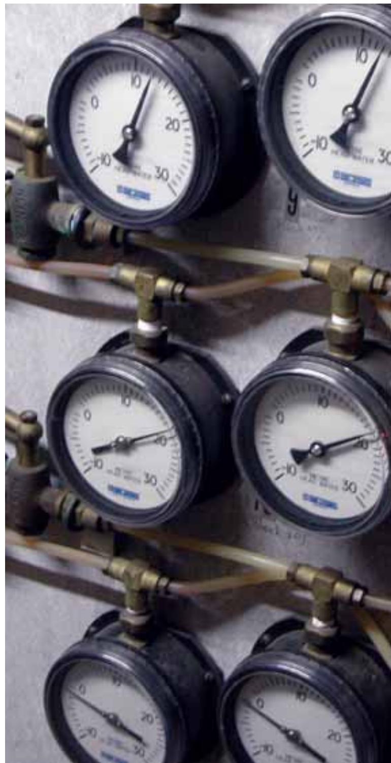
Piezometers are used to measure water pressure
