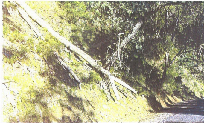
Fallen trees are common above the Road cuttings due to a combination of steeply inclined rock and road wash cuts. The Proposal is required in order to stabilise the cuts and to reduce the risk of trees falling onto the road.
