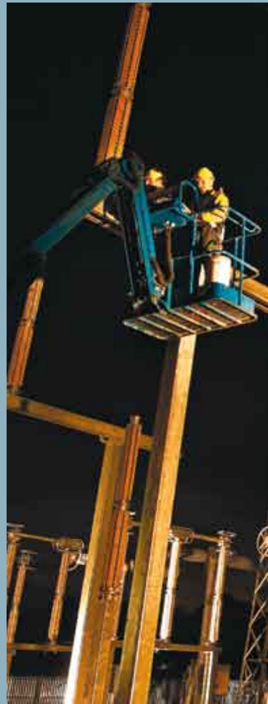
Steve Adams and Warwick Driez working on the construction of the Coffs Harbour substation
