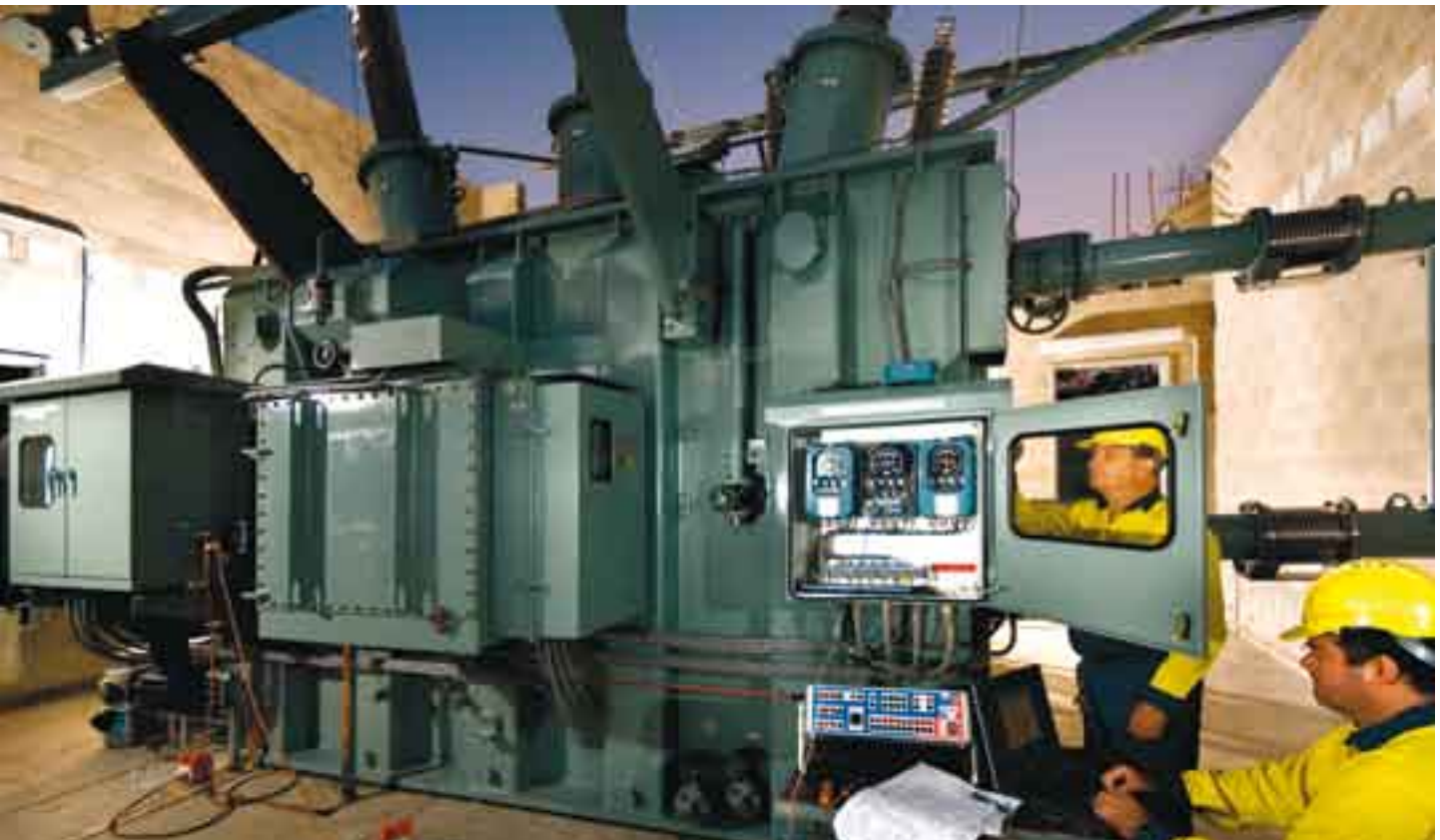
Graham McIlveen and Nick Osborne testing the newly installed Transformer at Port Macquarie Substation
